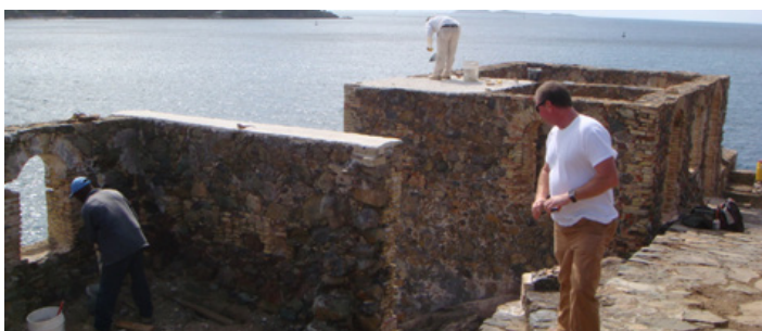
Masons working on Prince Frederiks Battery to cap walls and replace missing bricks and mortar.
